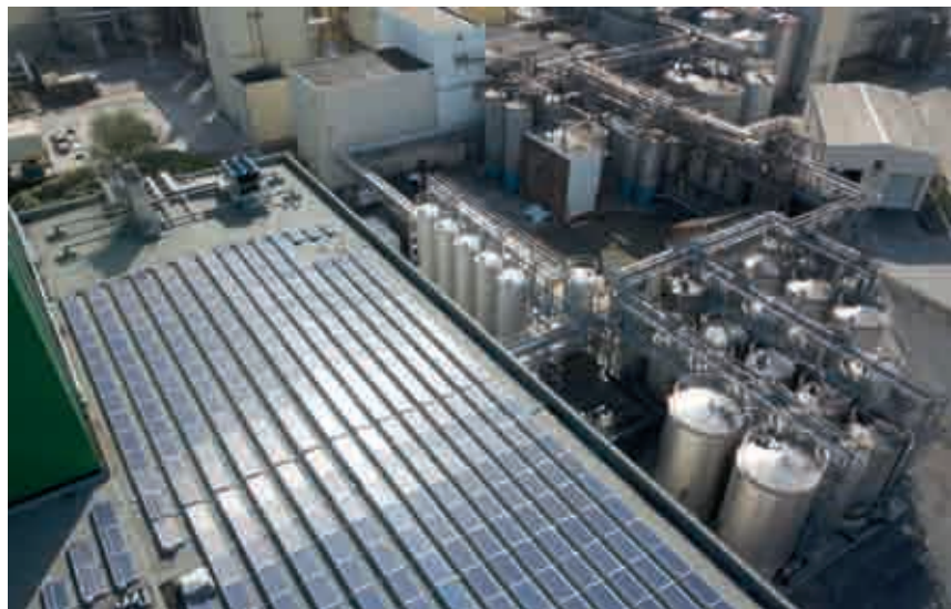
SOLAR PANELS ON THE ROOF OF THE PLANT.
