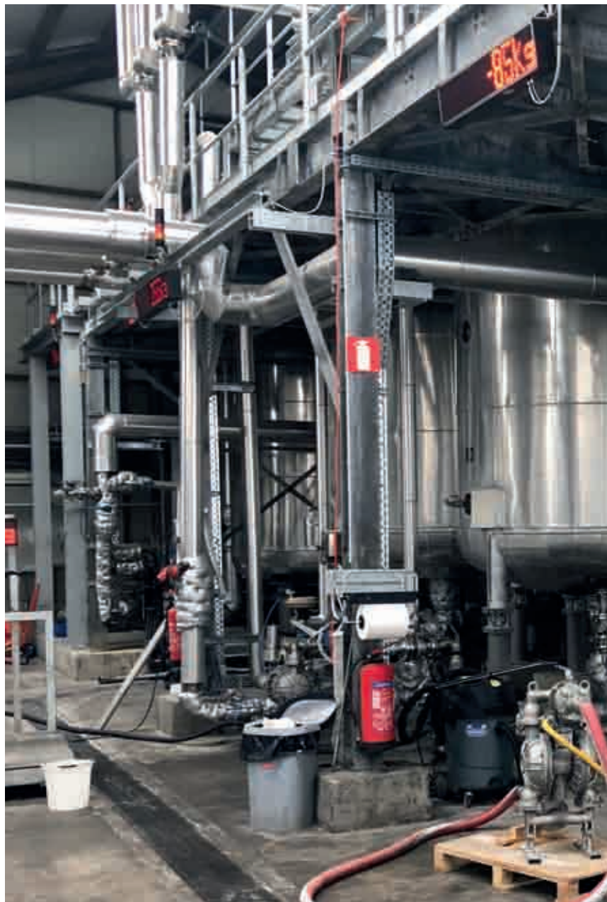
THERE ARE THREE 15M 3 STAINLESS STEEL REACTORS AND ONE 10M 3 HEAVY DUTY REACTOR AVAILABLE.
