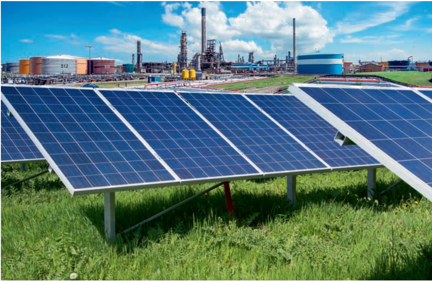
THE MORE THAN 28,000 HIGH-YIELD SOLAR PANELS WILL GENERATE AROUND 12.5MWH ON A SUNNY DAY.
