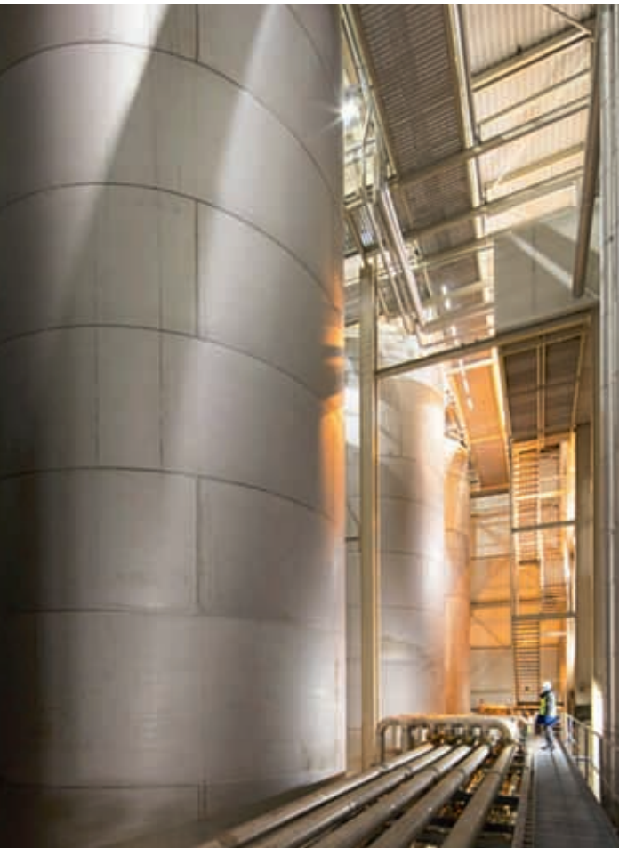
THROUGH A CLOSED CIRCUIT, THE JUICE IS PUMPED FROM THE VESSEL INTO THE 20M HIGH SILOS.
