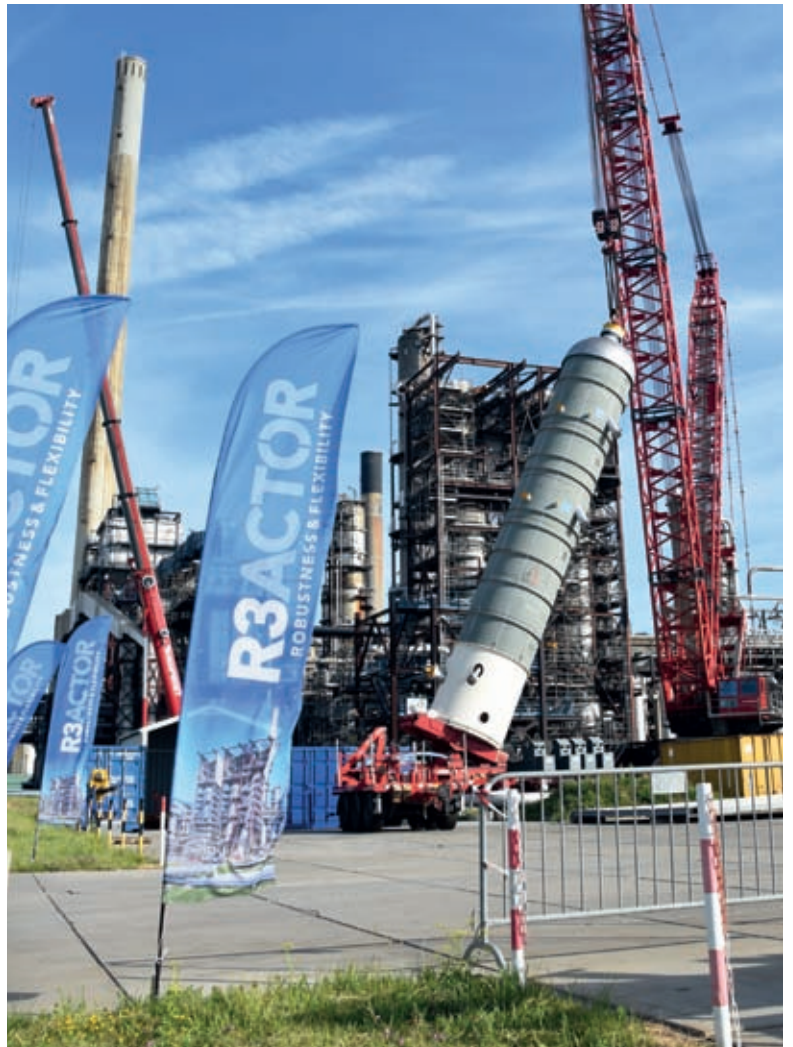
A GIANT CRANE HOISTS THE 600T REACTOR INTO AN UPRIGHT POSITION. IN THE FOREGROUND: CUSTOMISED BANNERS WITH THE REACTOR'S NAME AND SLOGAN.
