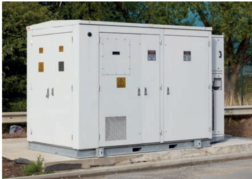
BATTERY STORAGE SYSTEM AT THE LANGERBRUGGEKAAL.
