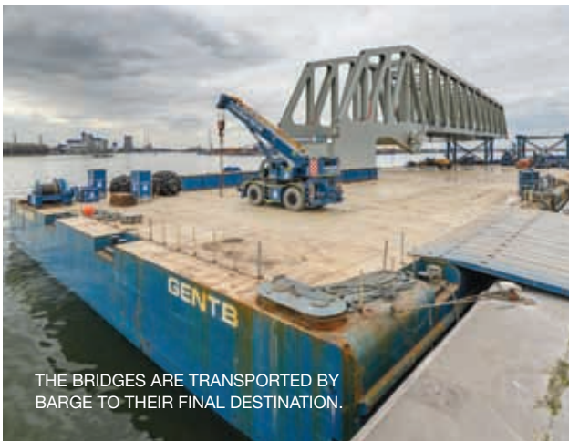
ONE OF THE TWO STEEL BRIDGES BUILT BY AELTERMAN FOR THE KIELDRECHTSLUIS IN ANTWERP.
