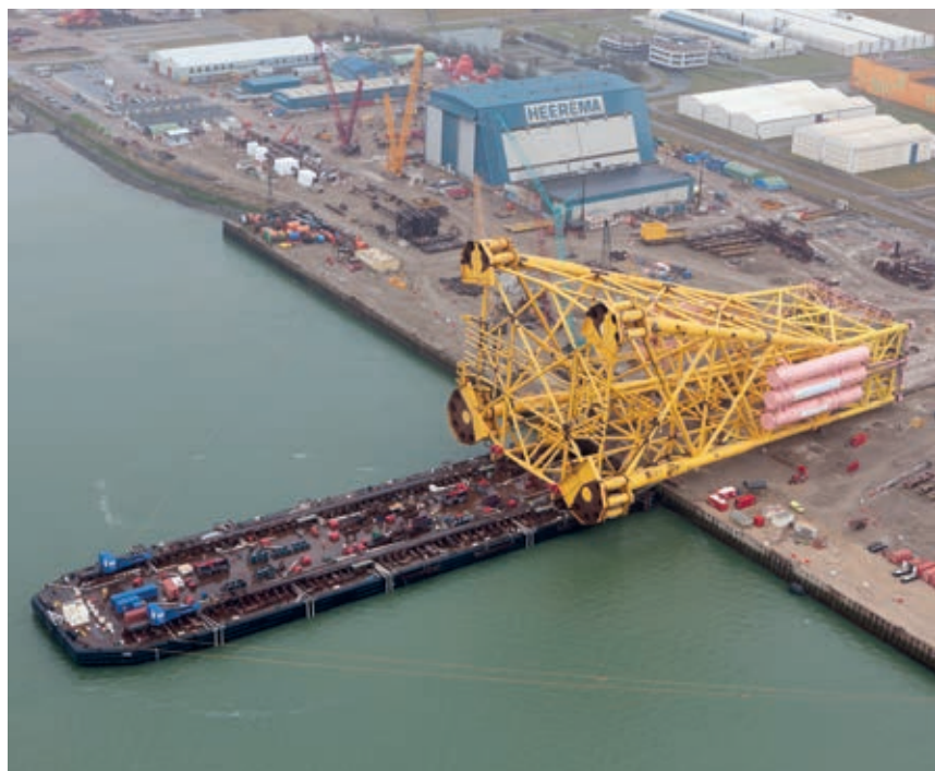
Load-out of the Gina Krog jacket in 2015. With its 17,000t, the jacket that Heerema constructed for Equinor really was huge.
