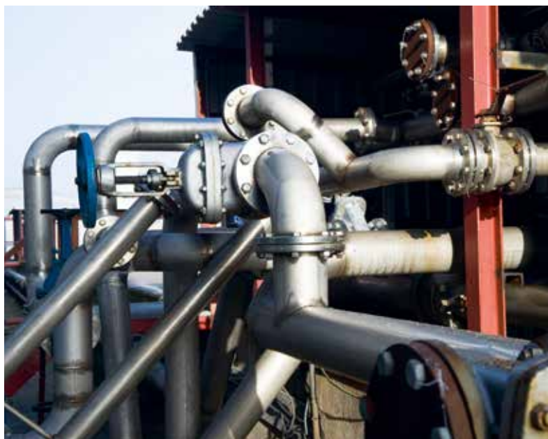
A dense network of pipelines will be of vital interest.
