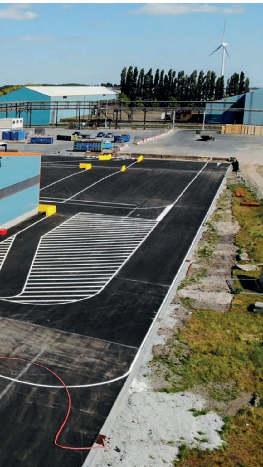
Molymet started building the new PurOx plant in 2017. It is now almost ready to start production.
