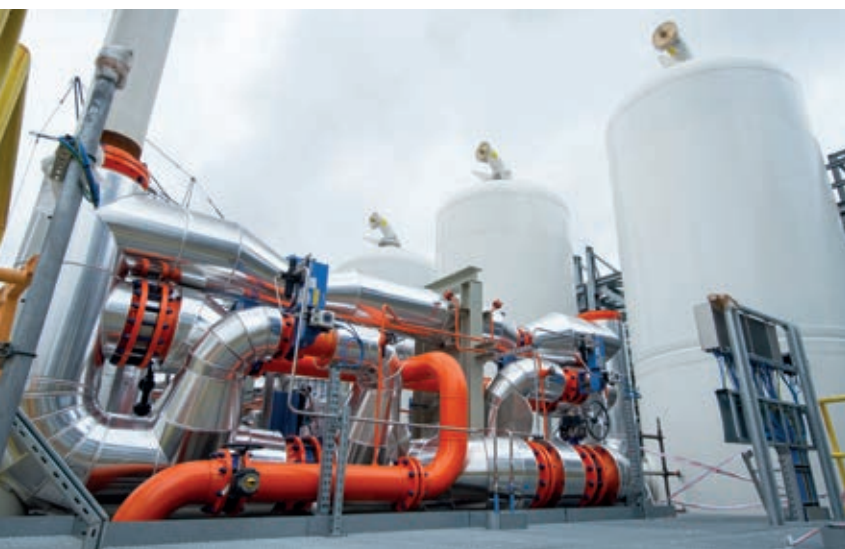
The Steelanol plant under construction. Steel and chemistry now go hand in hand.
