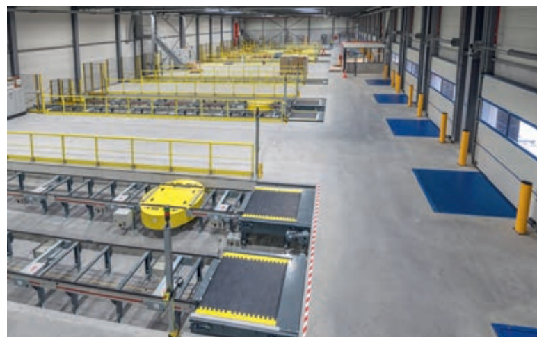
Pallets enter the expedition zone via conveyor belts, after which they will be loaded into the trucks
