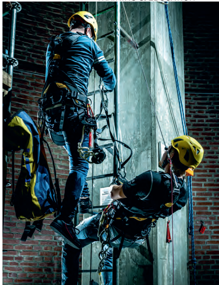
To work on the installation of TPs on monopiles, additional training is needed, such as for working at height.
