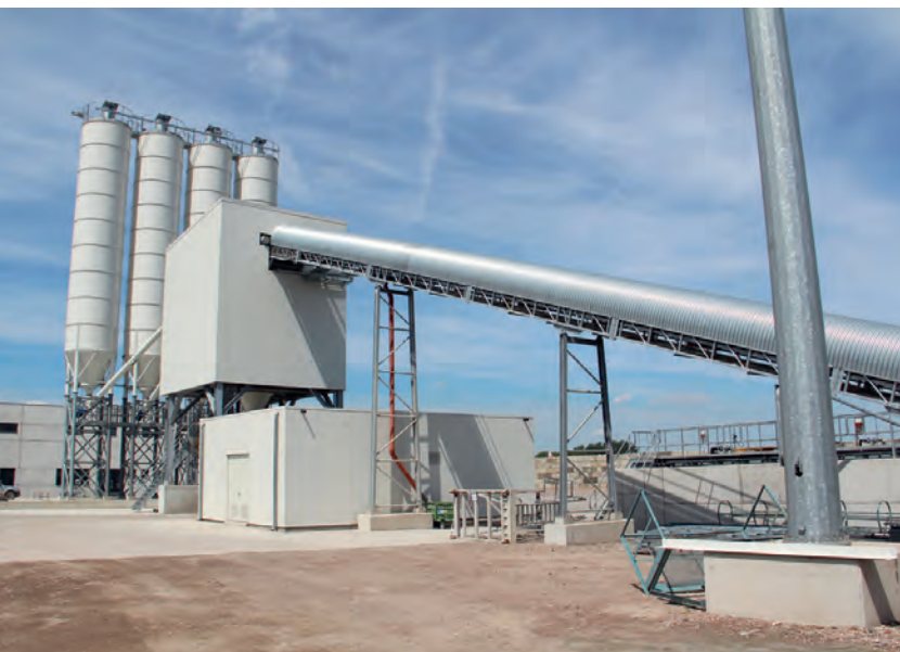
The new mixing plant can produce an increased number of varieties of concrete, including higher-grade ones for certified applications.
