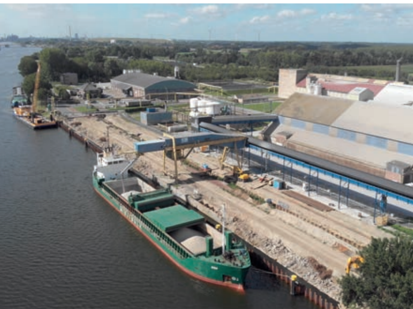
The Westkade in Sas van Gent was renovated whilst the terminal of Rosier/Borealis stayed operational.
