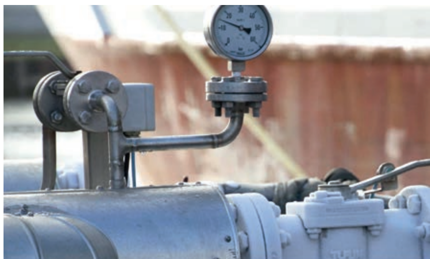
Detail of the existing loading installation at Yara Sluiskil. The cold liquid CO 2 is transported by vessel to the CO 2 reception installation in Øygarden, located on the west coast of Norway.
